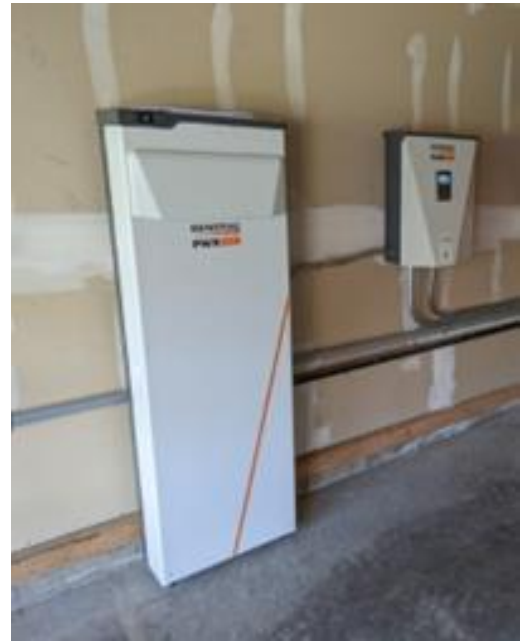
Fig 1: Generac PWRCell Battery and inverter.
